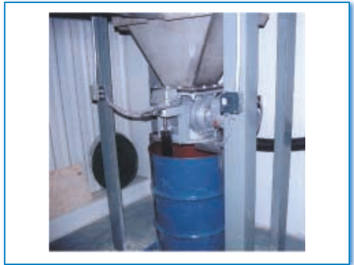
Ventilated Dust Container with Automatic Controls Located under the dust collector
