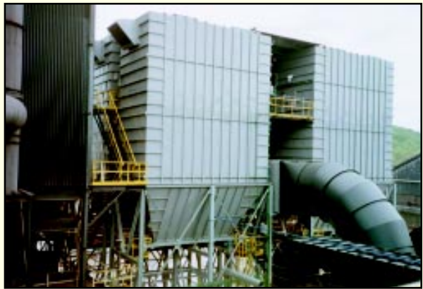
Primary and secondary emissions from an AOD vessel
