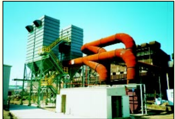
Ventilation for two 43-ton ladle metallurgy stations
