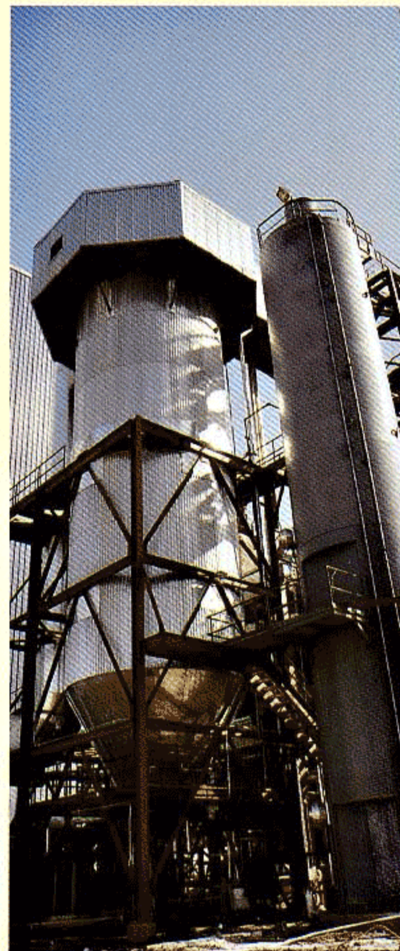
SO 2 and fly ash emissions from the 250,000 lbs./hr. pulverized coal fired boiler at this paper board plant are controlled by Wheelabrator spray dryer scrubbing and JET® III fabric filter technology.
